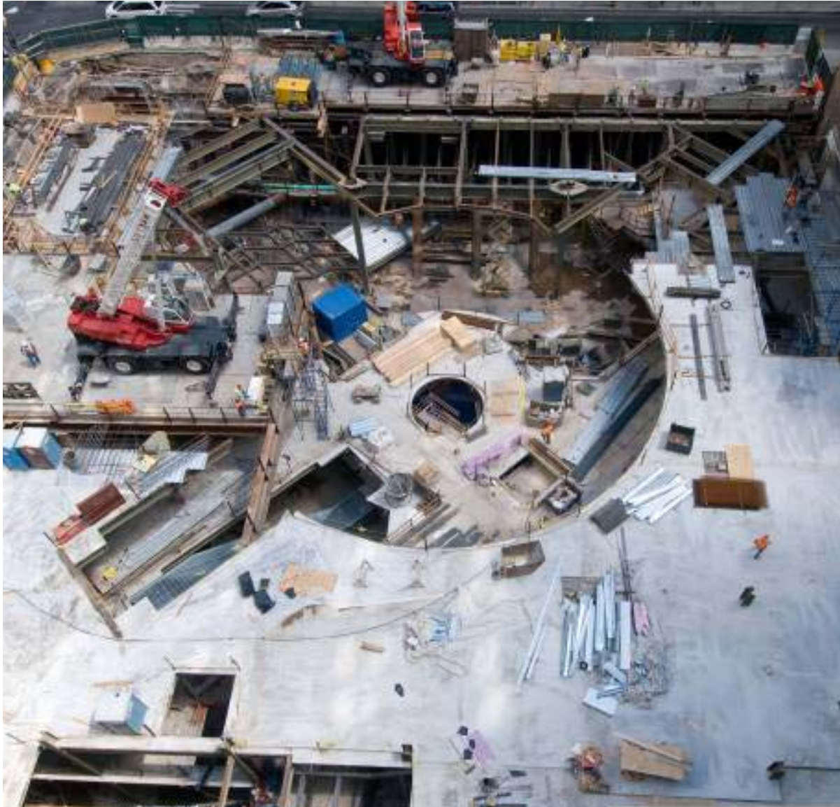
Aerial View of the Fulton Street Transit Center – North from Corbin Building
