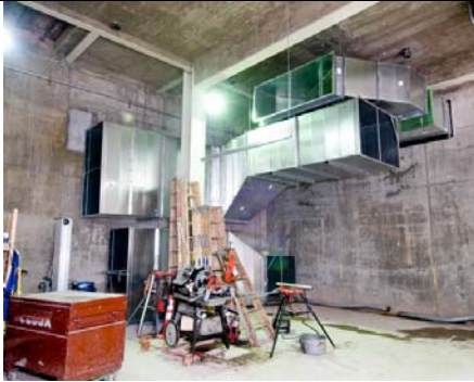
Concourse Level Utility Room Ductwork
